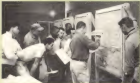
Job trainees in New York learn how to plaster a wall in 1965
